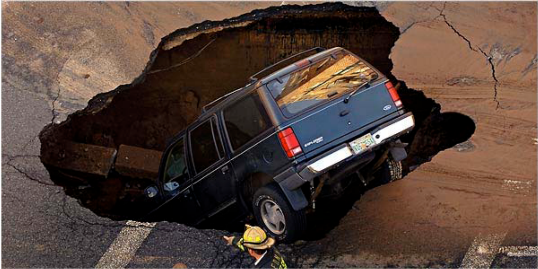
Result of a water main break, Portland, Oregon
